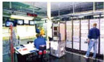
Industrial processes; programmable logic controllers, speed control processors, etc.
